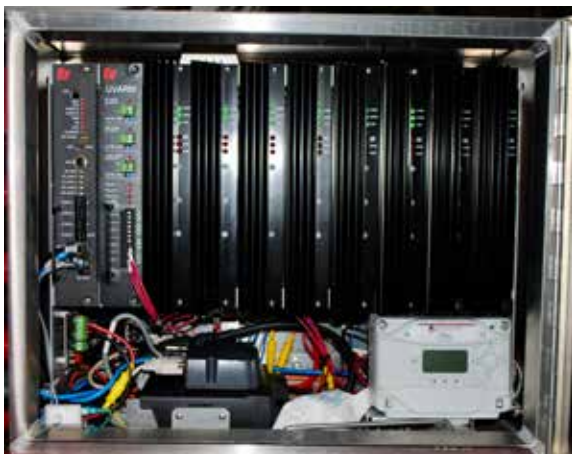
Figure 9 UVTD Control Cabinet
