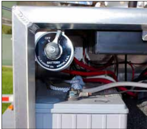
Figure 45 Siren master switch on
