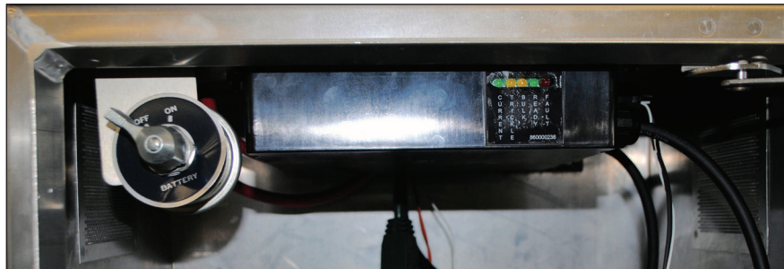
Figure 10 Mount the new charger with the disconnect switch
