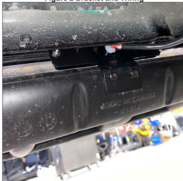
Figure 2 Bracket and Wiring
